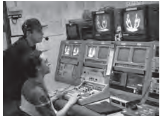
Television Control Room
